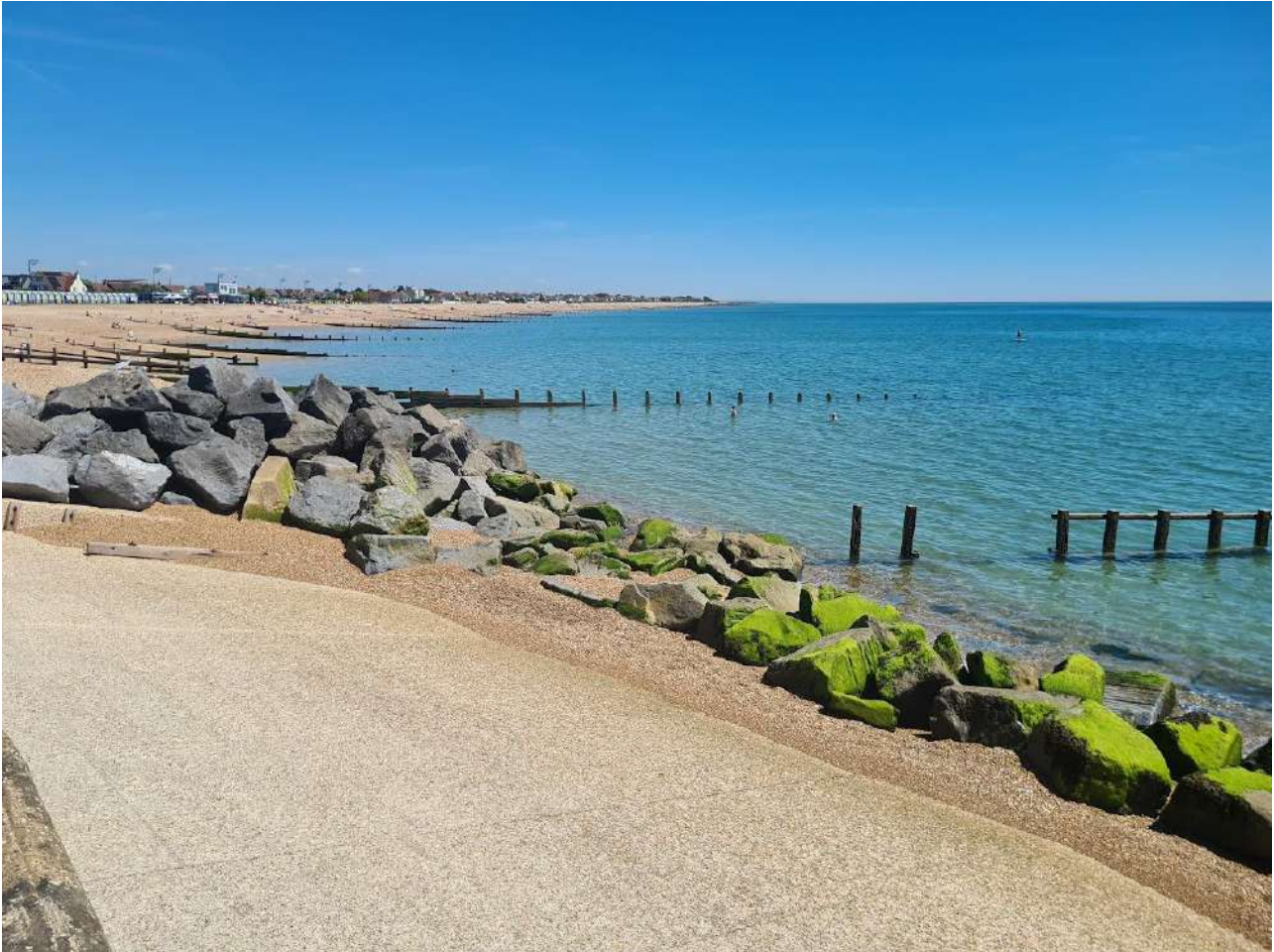
Figure 7: Groynes and rock armour along the beach in Bognor Regis. Source: author’s collection.
